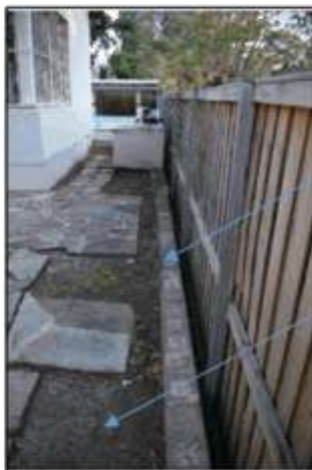
Figure 21. View to south-western boundary of site. Note the retaining wall suggesting that levels have been altered. Possibly at the same time as the rear addition (Source: Micris Design, June 2020).
