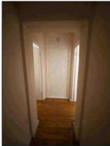
Figure 23. Internal view to dwelling within the rear. Note different timber flooring and the width of the wall in between.
