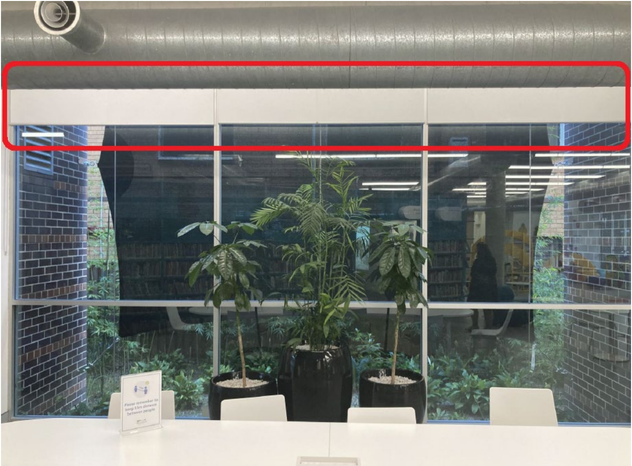
Figure 12. Image of the windows on the library's southern elevation showing the shade screen installed outside and the blinds outlined.
