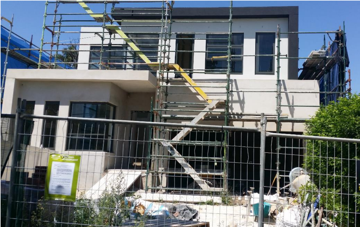
Figure 2: Streetscape view of subject site and dwelling under construction from Myrna Road
